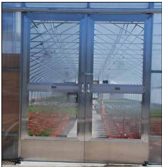
Double sliding doors with clear vision glass panels.
