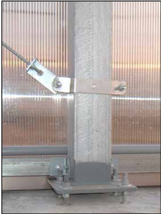
This photo shows a column with a base plate mounted on a concrete wall.
